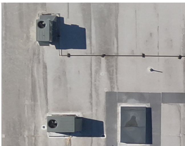
HVAC Equipment Area 1
