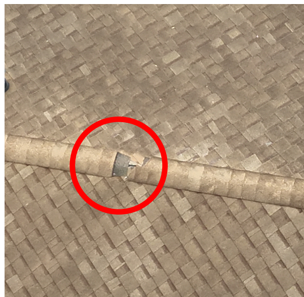
Close-Up of Missing Shingle Area
