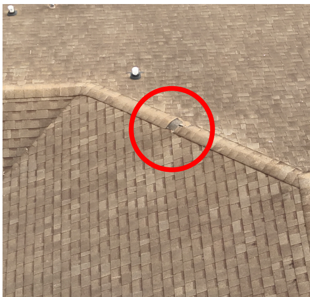
Overall View of Missing Shingle Area
