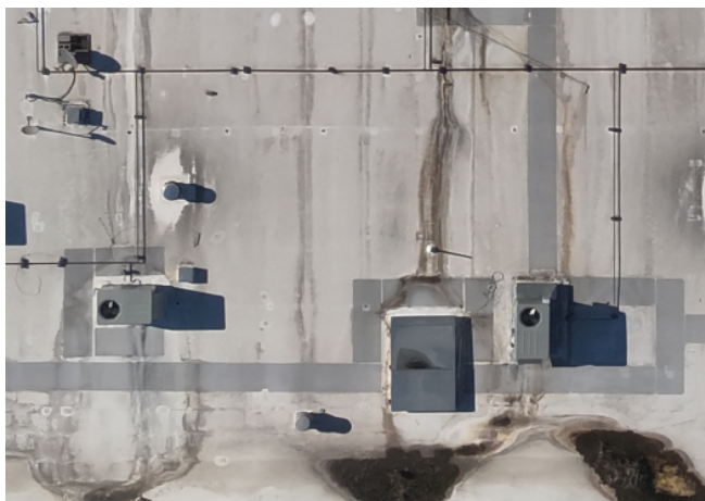
HVAC Equipment Area 3
