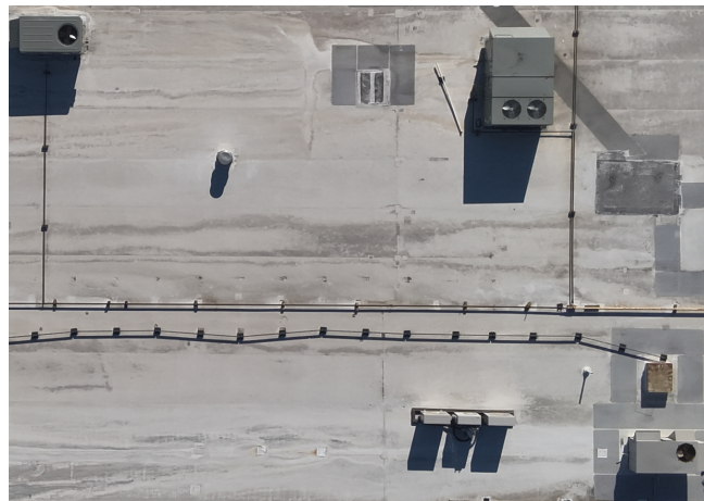
HVAC Equipment Area 4
