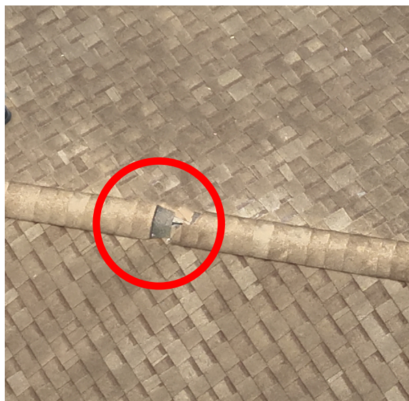
Close-Up of Missing Shingle Area
