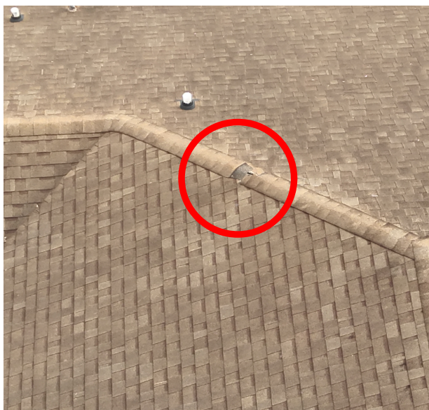
Overall View of Missing Shingle Area
